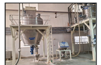
PNEUMATIC CONVEYING SYSTEMS
