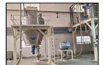
PNEUMATIC CONVEYING SYSTEMS
