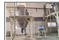
PNEUMATIC CONVEYING SYSTEMS
