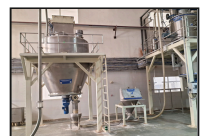
PNEUMATIC CONVEYING SYSTEMS
